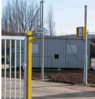
Site entry with transponder card reader system
